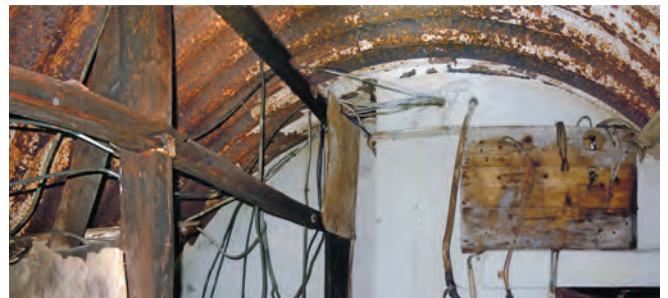
Cable Distribution Panel
